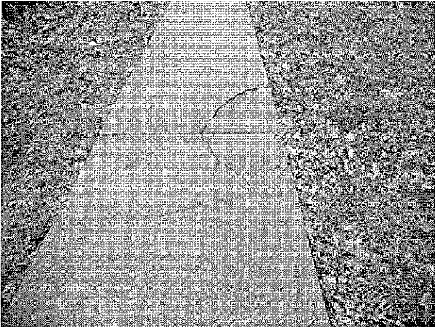
A9 _Cracked Walkway
