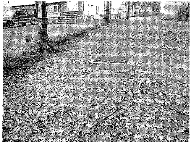
A12 _Raised Storm Drain Inlet
