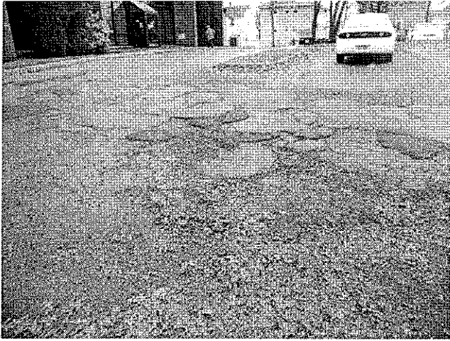
A1 _Asphalt Surface Defects
